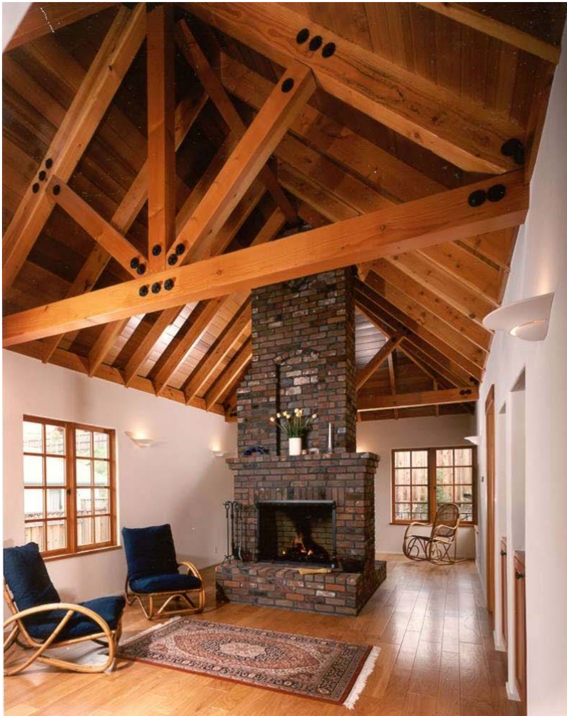
A rebuilt and better version of the chimney rises through the middle of the living room with no adjacent walls. Photo: Allen Geller
